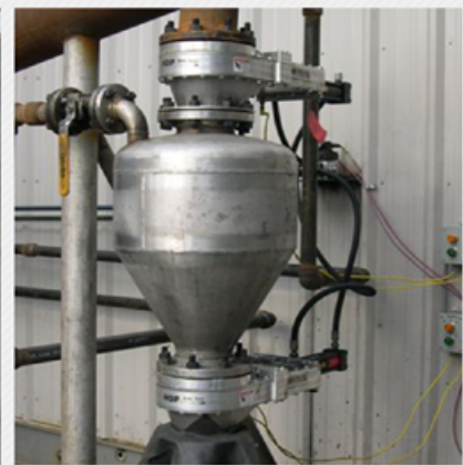
12" (305mm) HDP above and below a pressure pot handling PRB coal & wood chips
