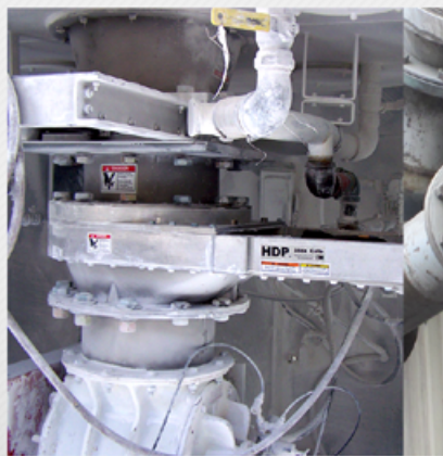
16" (406mm) HDP above an airlock handling calcium oxide
